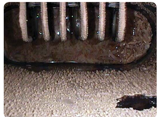
Scaled heating coils and boiler wall from a coffee brewer after 1,325 gallons of 25 grains per gallon untreated water.
